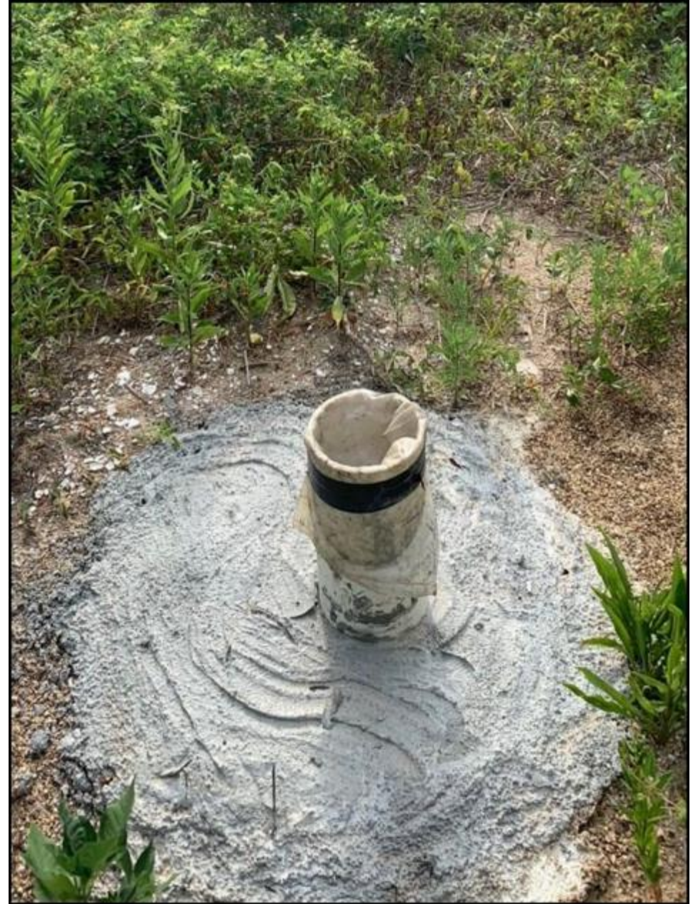
Example 18: Non-Compliant improper cap, plastic bag/liner, with no pump equipment installed
