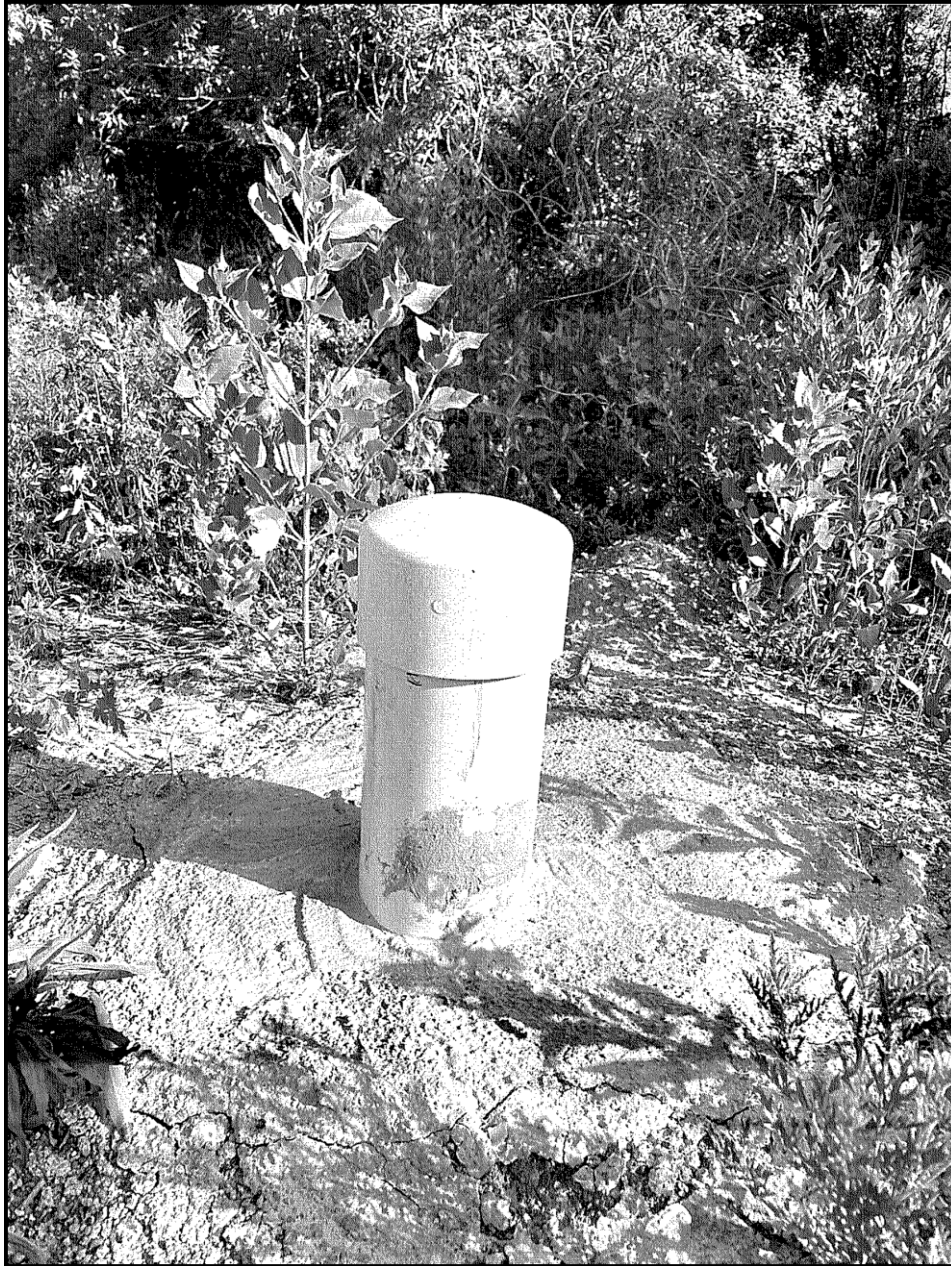
Example 17: Compliant properly capped well with no pump equipment installed
