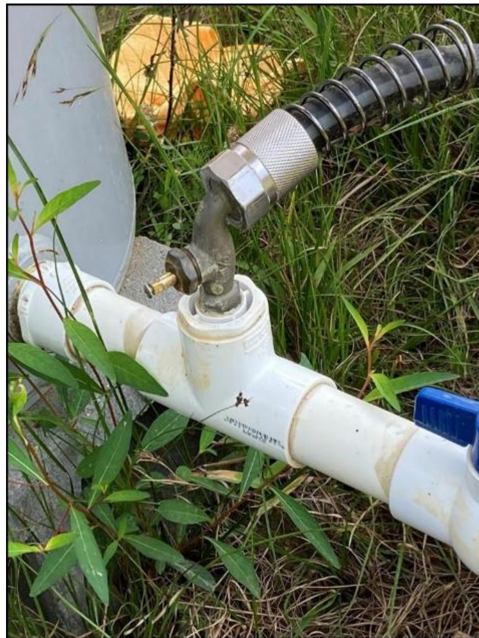
Example 14: Non-Compliant threaded nozzle and not sampling tap not turned downward
