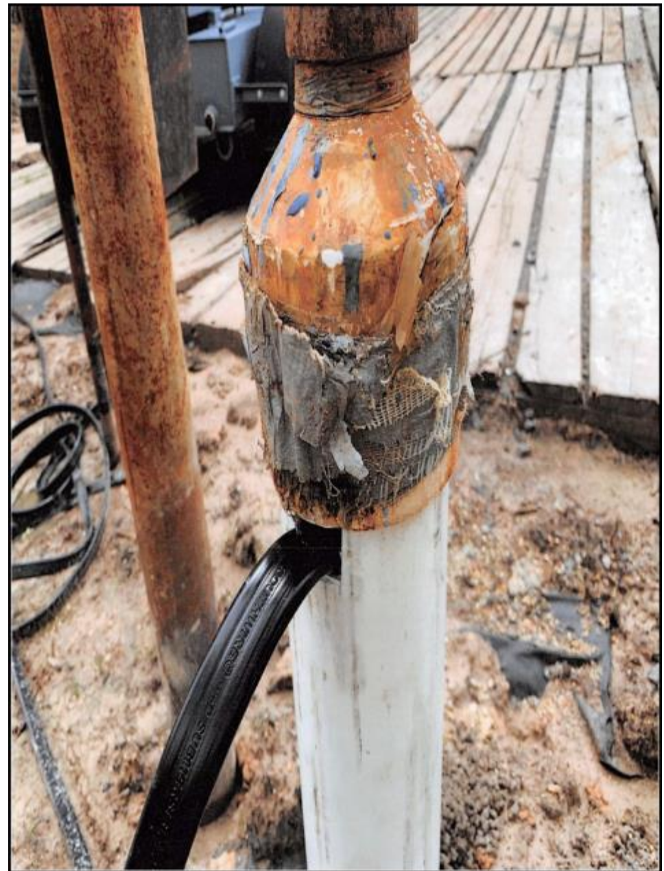
Example 10: Non-Compliant improper sanitary seal, not watertight
