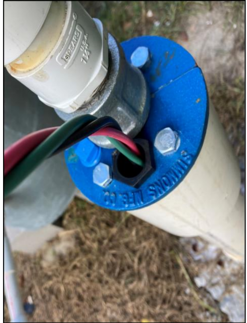
Example 8: Non-Compliant wire entering the well, not watertight
