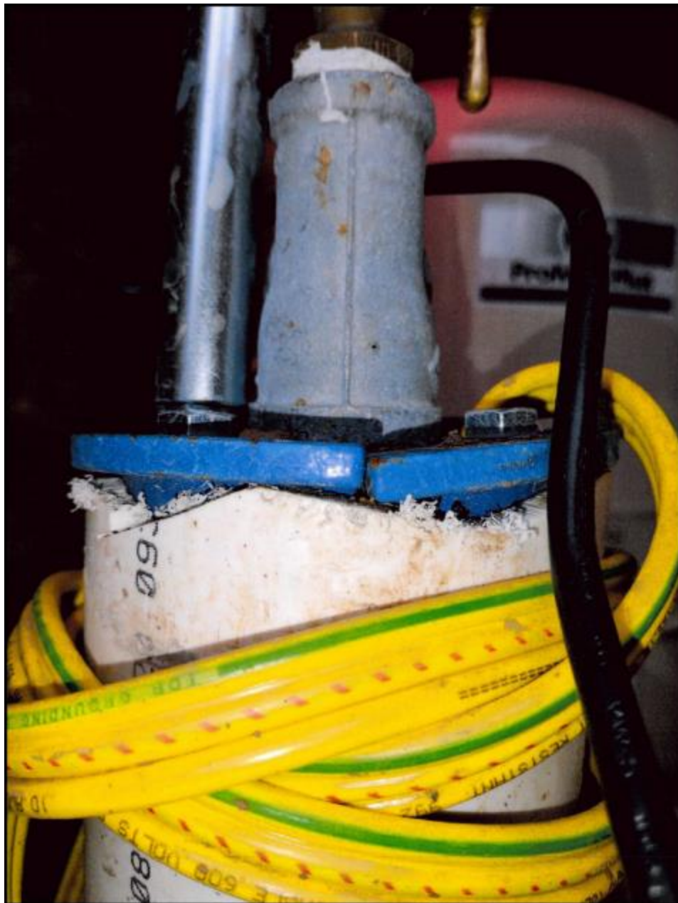
Example 9: Non-Compliant sanitary seal not watertight, casing not flush
