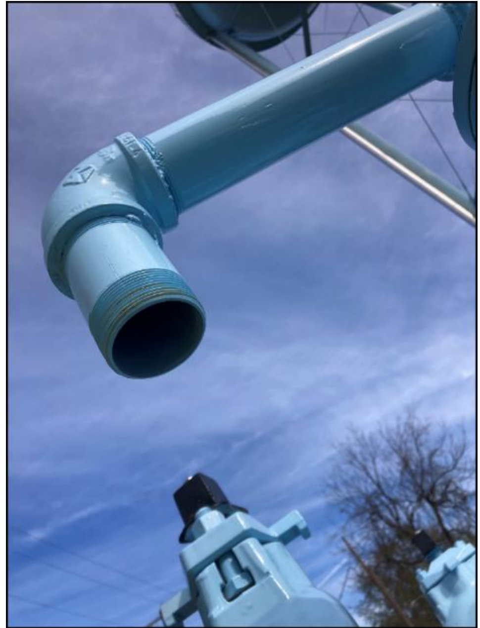
Example 12: Non-Compliant vent is not screened
