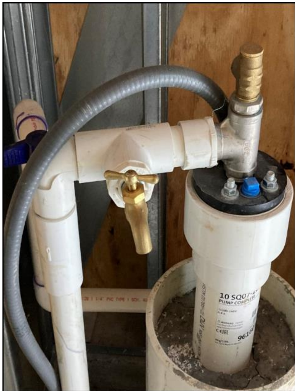
Example 13: Compliant smooth nozzle type sampling tap turned downward
