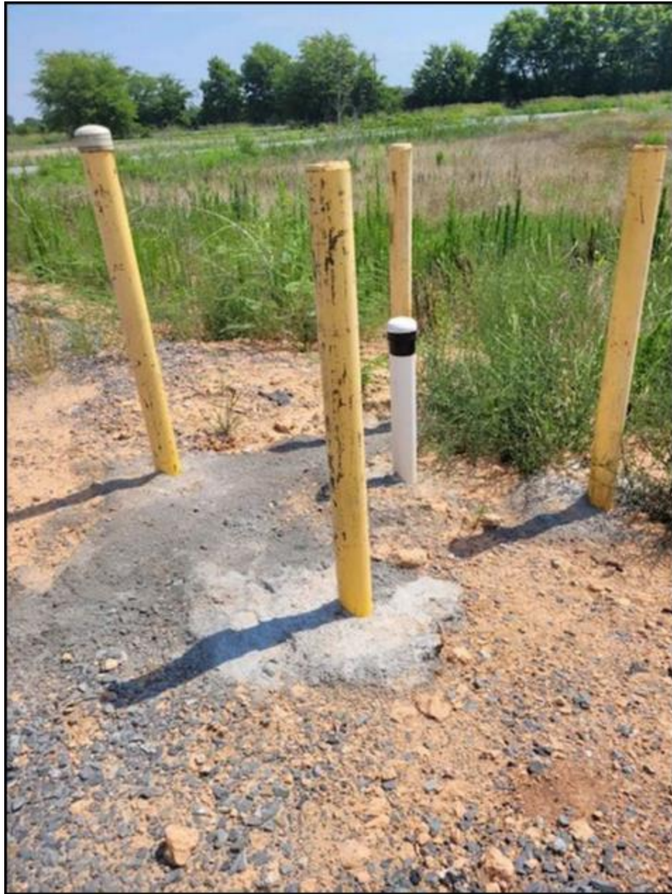
Example 15: Compliant four corner posts cemented to ground surface
