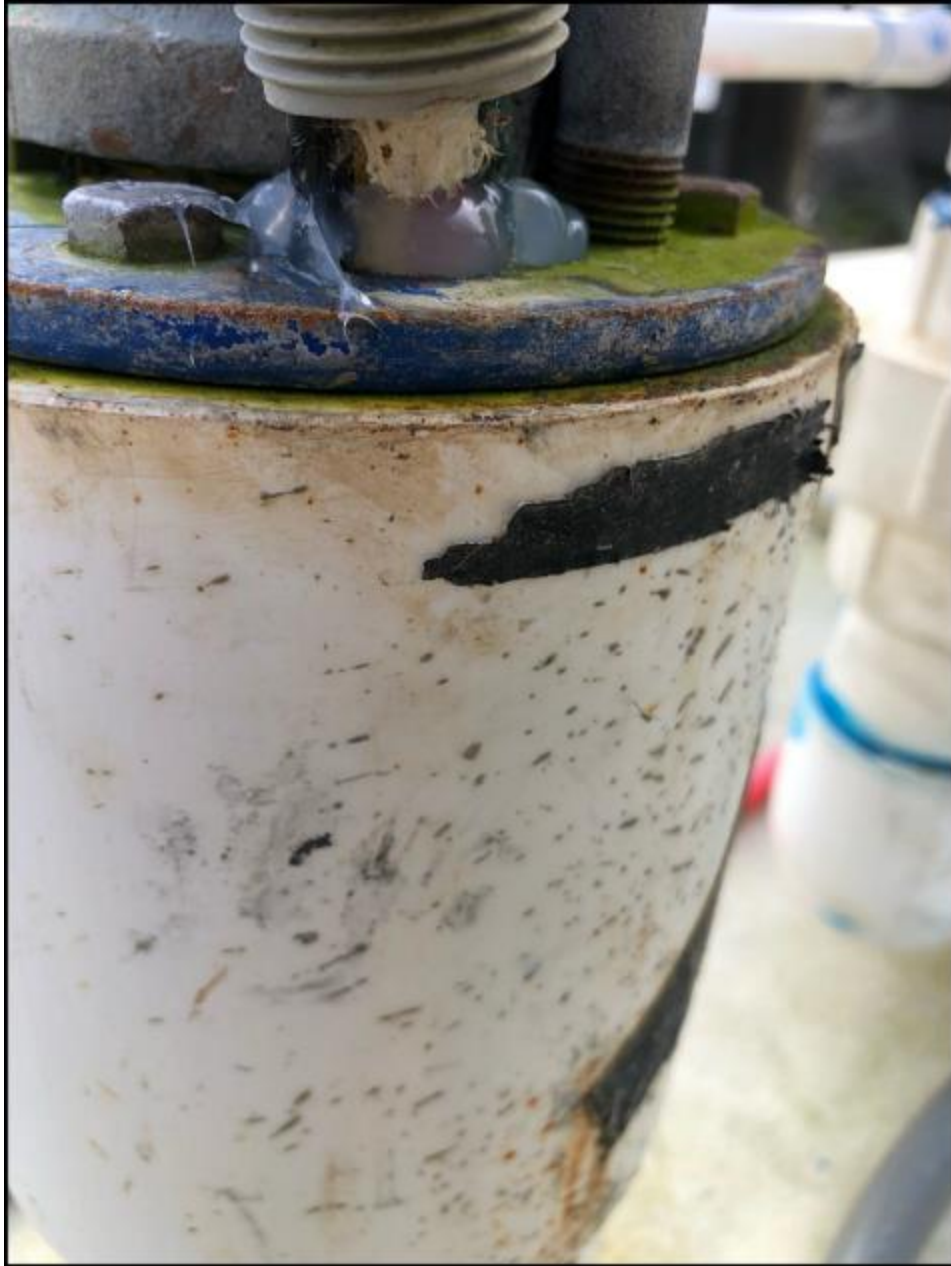
Example 7 Compliant properly installed sanitary seal
