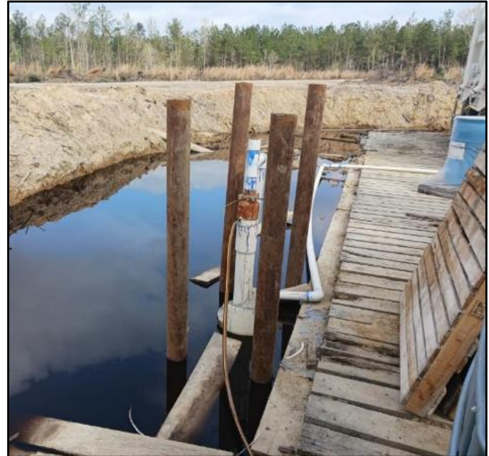
Example 20: Non-Compliant, installed in water
