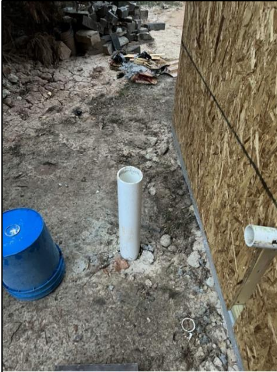
Example 19: Non-Compliant, no cap on well with no pumping equipment installed. *See Example 17 for a properly capped well with no pumping equipment.
