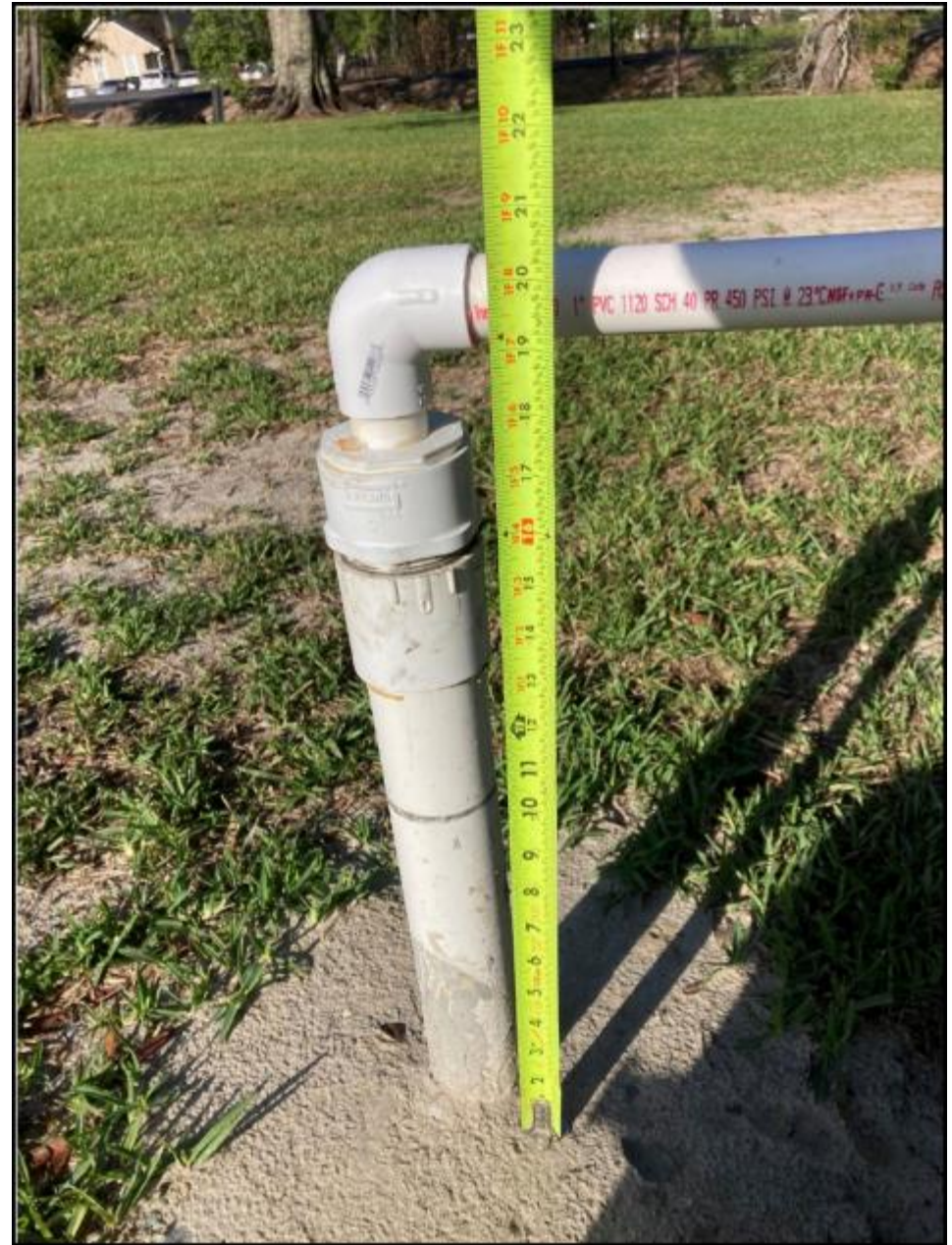
Example 2: Non-Compliant casing height less than 2 feet
